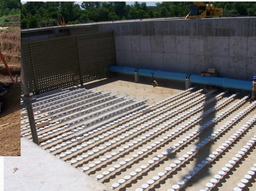
New Aeration Basin #3
